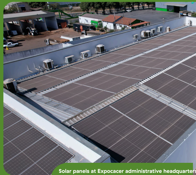
Solar panels at Expocacer administrative headquarters
